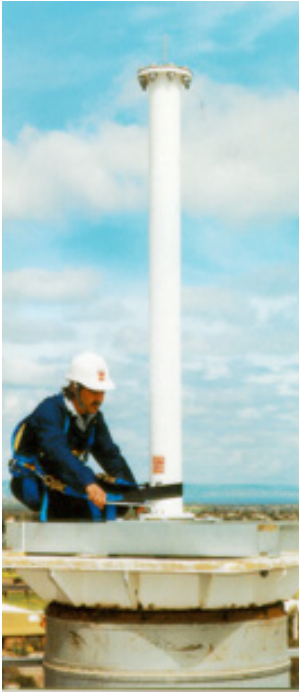
Fig. 4: Final touches to the alignment of AV channel diplexers in a 19 channel SOW MMDS headend installation. The headend is one of 12 supplied by RFS Australia to pay television company - Austar.
