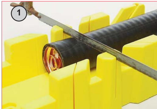
Straighten cable and ensure that it is marked and cut square using a mitre box or similar aid.
