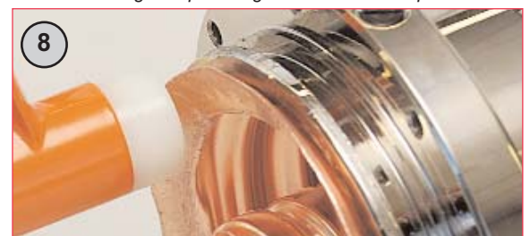
8 Remove PVC tape and finish flaring process with the nylon hammer taking extreme care not to split or break the copper outer conductor (refer Step 15 for remedial process).
