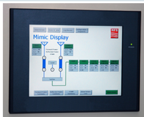
MSV2 System monitor
